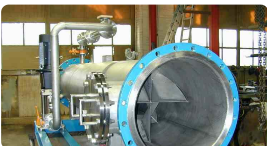
CO 2 feeding via side stream into the main water stream
