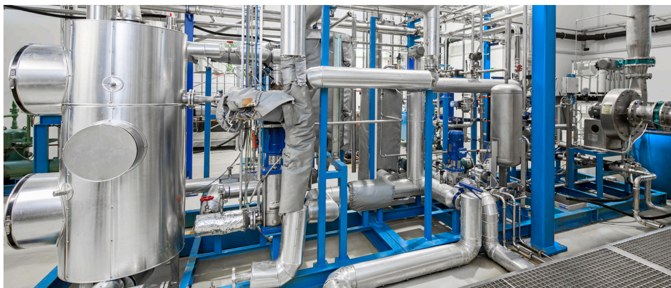
Process unit with reboiler
