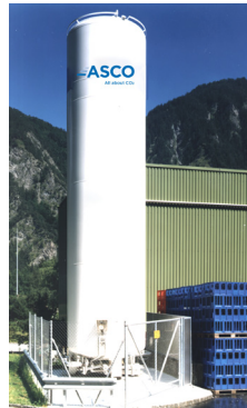
Vertical CO 2 storage tank
