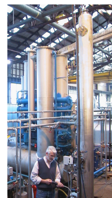
High pressure purifier
