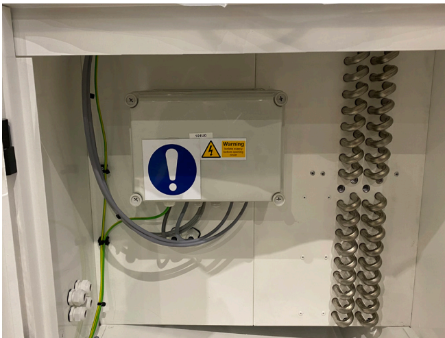
Terminal box for external control cabinet
