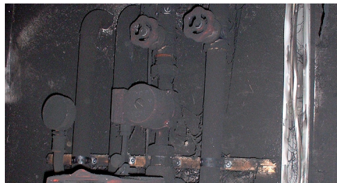
Fire damage before ...
