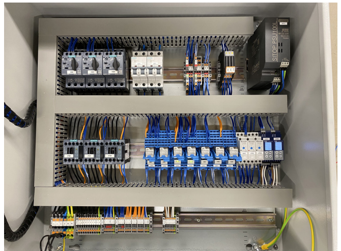
External control cabinet with 10 m connecting cable, temperature sensors and cabinet heating
