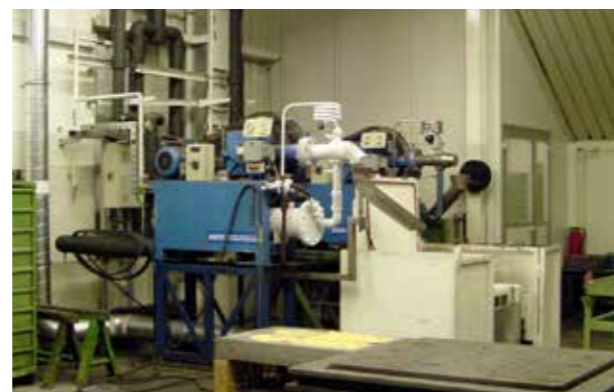
The in-house dry ice production provides an increase of flexibility and quality in the daily working process.
