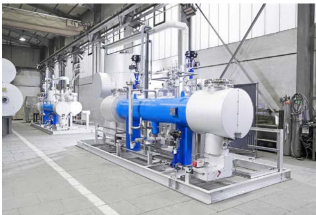
Figure 1 – ASCO CO 2 By-Product Recovery Plant
