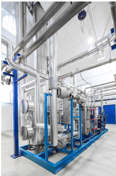
Picture 2 – 6.8 MTPD CO 2 Stack Gas Recovery Plant by ASCO
