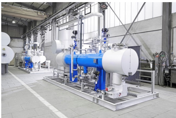
Figure 1 – ASCO CO 2 By-Product Recovery Plant
