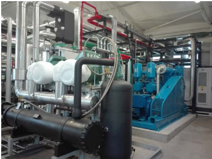
Picture 1 –ASCO CO 2 liquefaction plant (left) and ASCO CO 2 compressor station (right)
