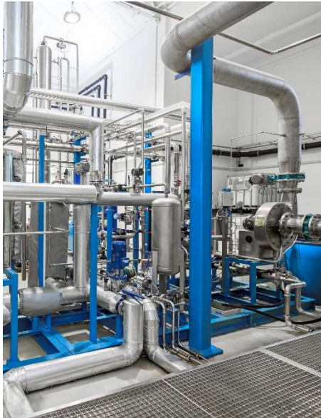
ASCO CO 2 Production Plant
