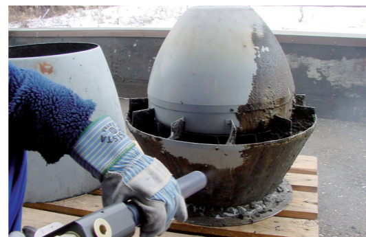
Cleaning of industrial fan
